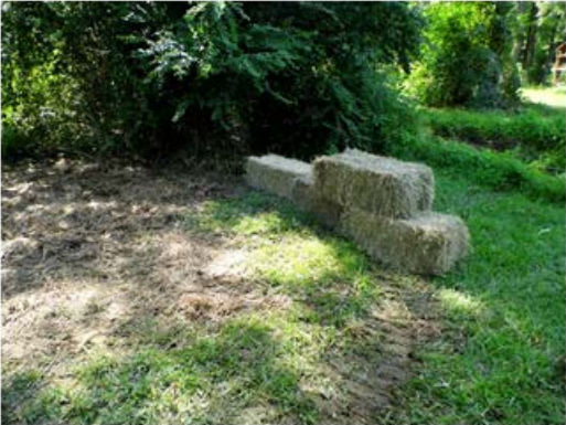
Storm water protection
